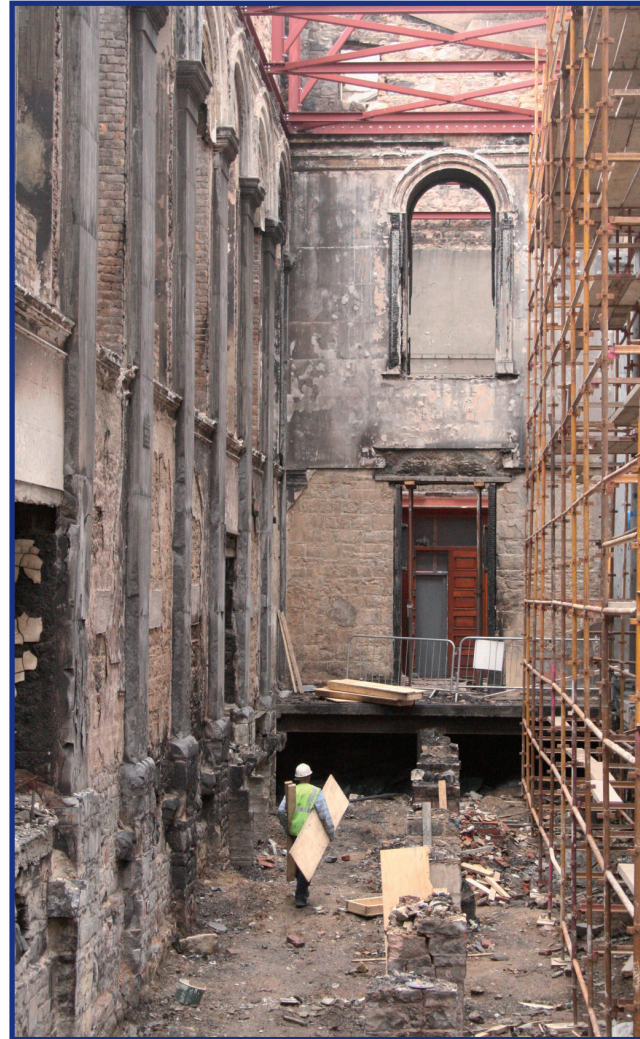
The extent of the damage to the right side aisle.
