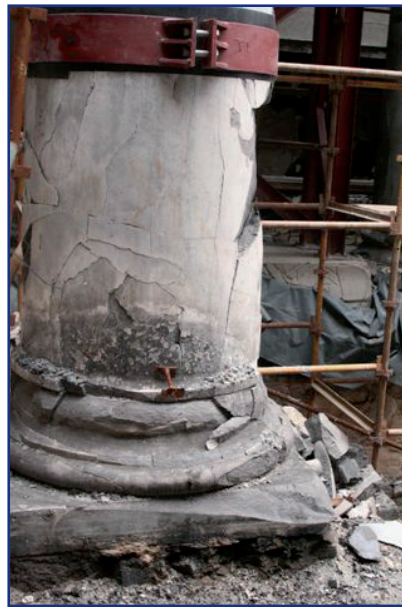
One of the damaged pillars.
