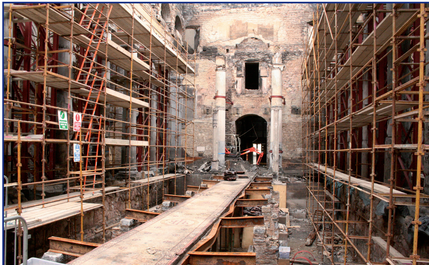
All that remains of the Cathedral floor is the fragile centre aisle.
