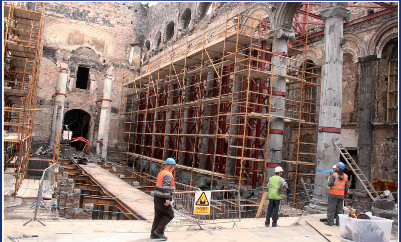
Extensive steelwork is put in place to safeguard the building as part of the emergency works.
