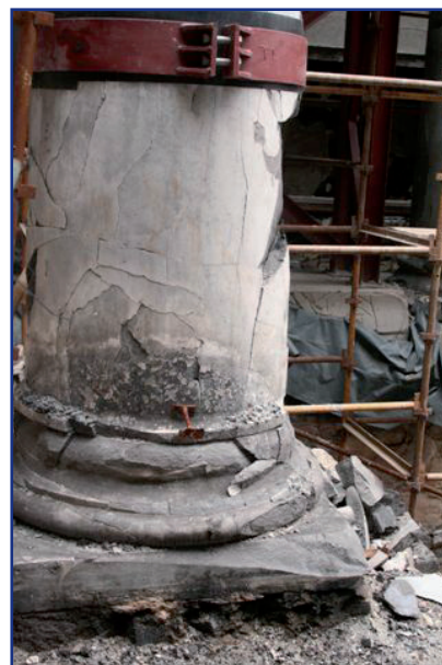
One of the damaged pillars.
